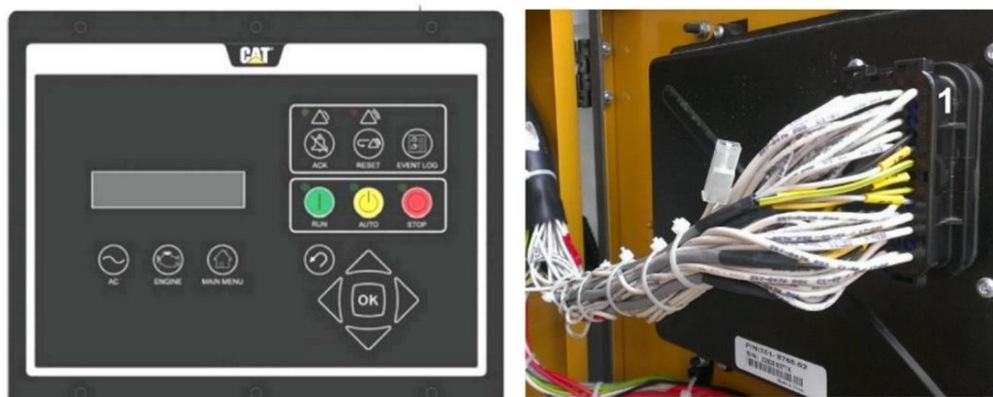
Figure18. Main controller of diesel generator
