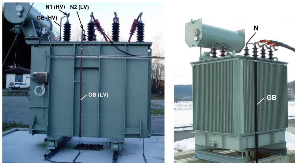
Figure 13: Power transformers with grounded neutral conductors N. GB – ground bus. LV – low voltage side; HV – high voltage side.
