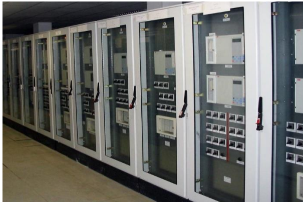
Figure 9: Cabinets with electronic equipment of supervision, automation and relay protection used in the power industry.
