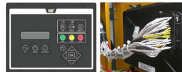
Figure 18 Central controller of diesel generator
