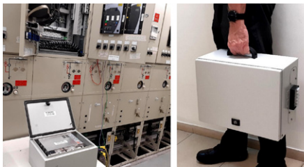
Figure 14 HEMP protected backup power supply for electronic equipment testing after HEMP impact
