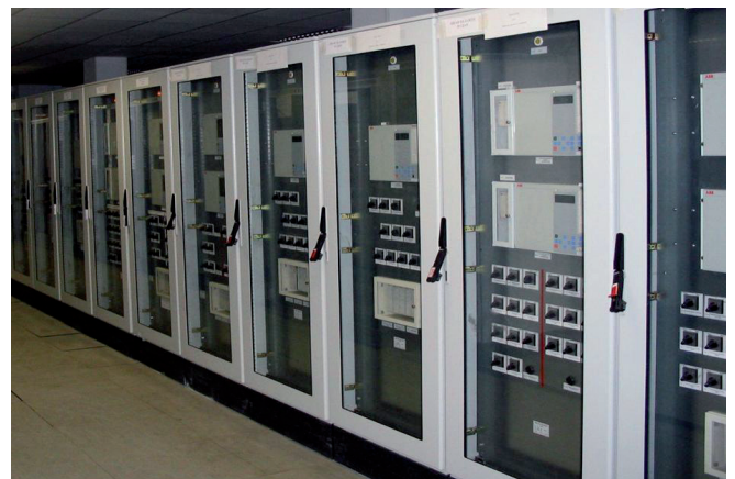
Figure 4 Contemporary way of electronic equipment mounting in cabinets
