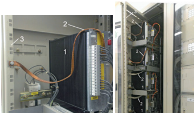
Figure 2 Arrangement of DPR multipoint grounding with equipotential plane 1 – DPR in metal casings; 2 – bounding strip; 3 – metal cabinet's element that performs the role of the equipotential plane.
