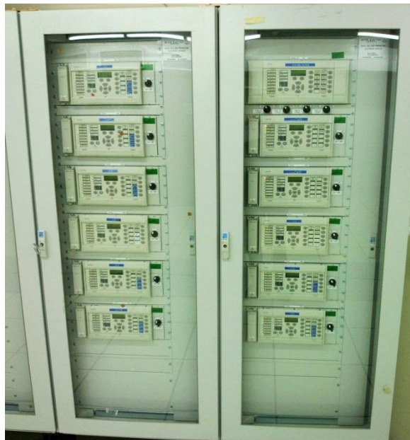
Fig7. Modern relay cabinets with glass doors
