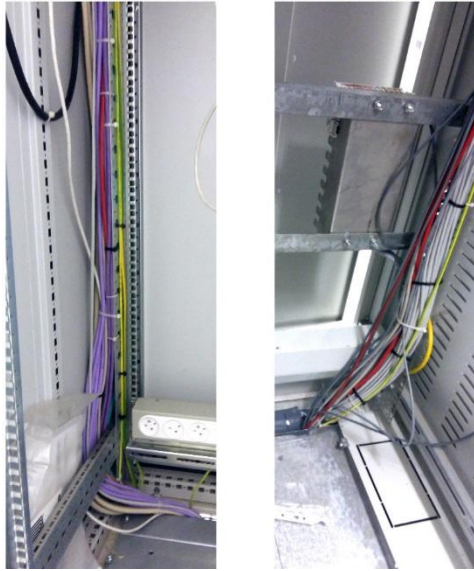
Fig. 6. Cable harnesses entering the communication cabinets through the floor opening
