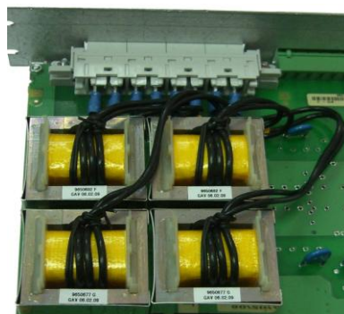
Fig6. Section of a module showing the analogue inputs of DPR with installed CT. You can clearly see the primary winding, which consists of 4 coils of flexible insulated black wire.
