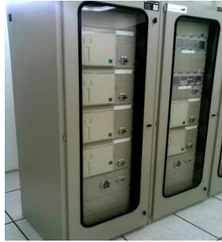
Fig5. DPR terminals installed in standard cabinets with glass doors
