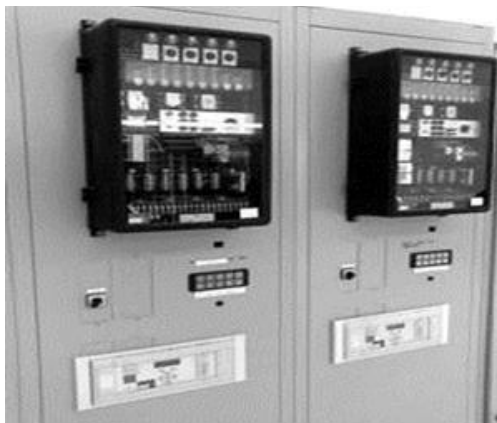
Figure 1 - Section of distance protection charge of 160 kV lines containing electromechanical relay of LZ31 type (top) included in the parallel operation with microprocessor protection of MiCOM P437 type
