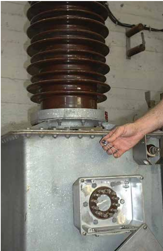
Technician prepares to connect the protection device (in hand) to the current transformer.
