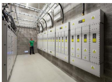
Figure6. HEMP filters manufactured by Euro-EMC (Great Britain) in a protected concrete shelter
